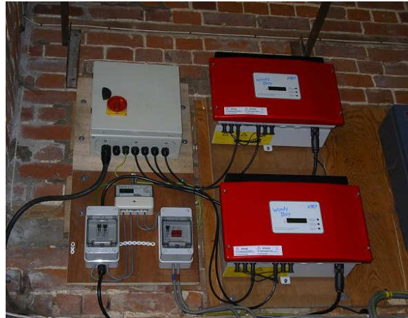
Above: Control panel and inverter units
